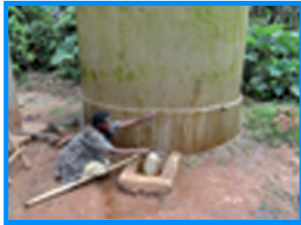
Household tank by ATC in Kikandwa model village placed on a raised platform and the tap placed in an accessible position.
