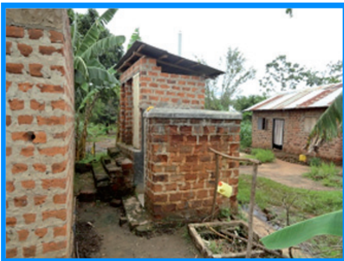
Household hanging toilet and bath shelter with barrier (step)
